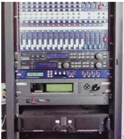
Rack detail. The feedback eliminator is no longer required.
